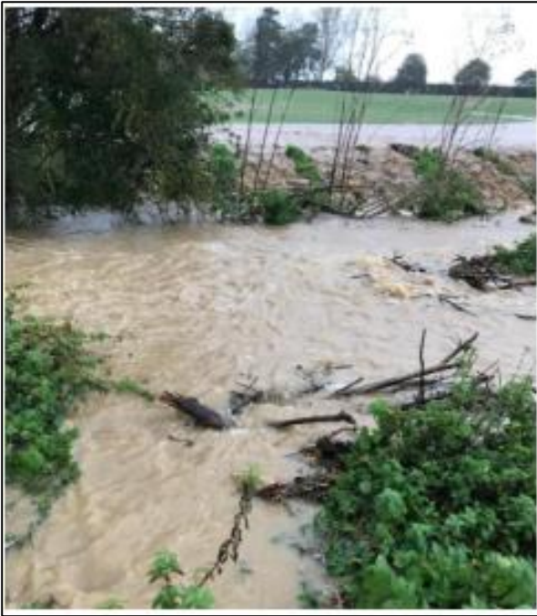
Photo 7: Ditch overflowing upstream of highway culvert opposite Garnetts Gardens.
