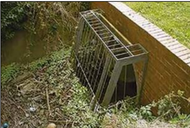
Photo 17: Trash screen example (CIRIA Culvert, Screen and Outfall Manual C786F)
