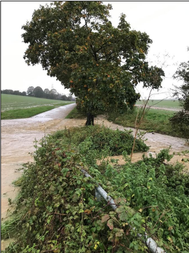
Photo 3: Exceedance of ditch capacity upstream of highway culvert opposite Garnetts Gardens
